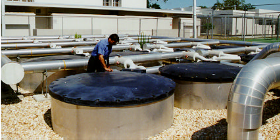
Ice storage tanks partially embedded in the ground.
