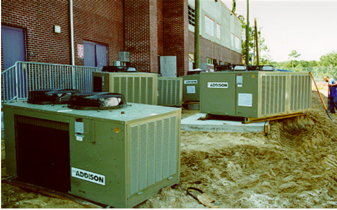
Condensing units for Split System
