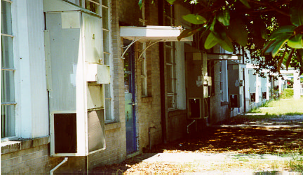
Array of Through-Wall units in elementary school
