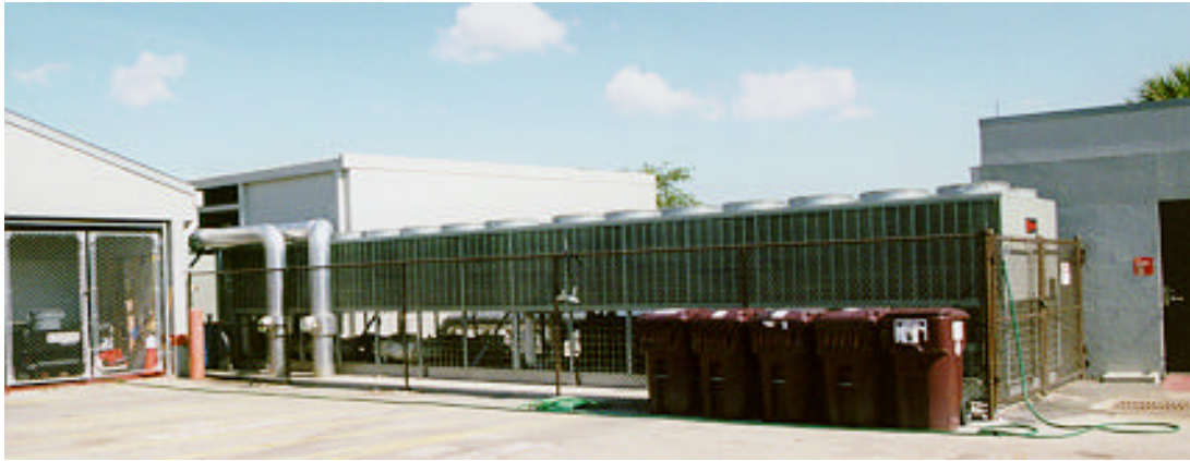
Air cooled chiller in equipment yard
