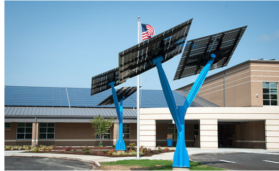
Spotlight Solar product “Lift” at net-zero school in NC, Sandy Grove Middle School
