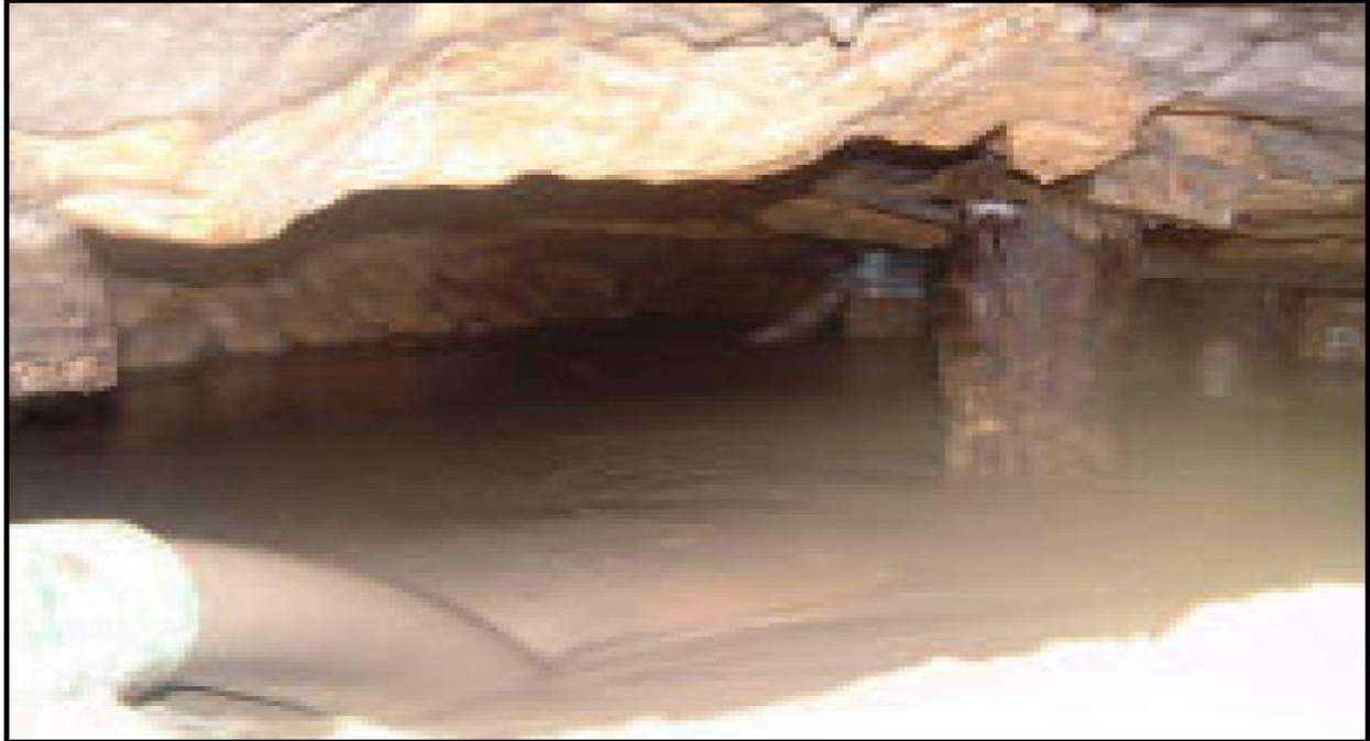
Figure 1.2 Large scale LFC infilling of an old mine in Combe Down, United Kingdom.
