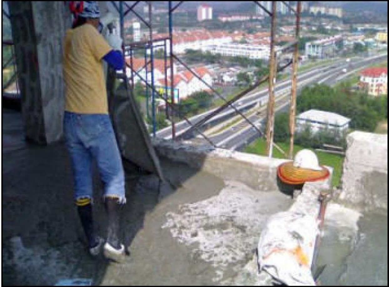
Figure 1.4 LFC being employed in a high rise building floor screed in Penang, Malaysia.
