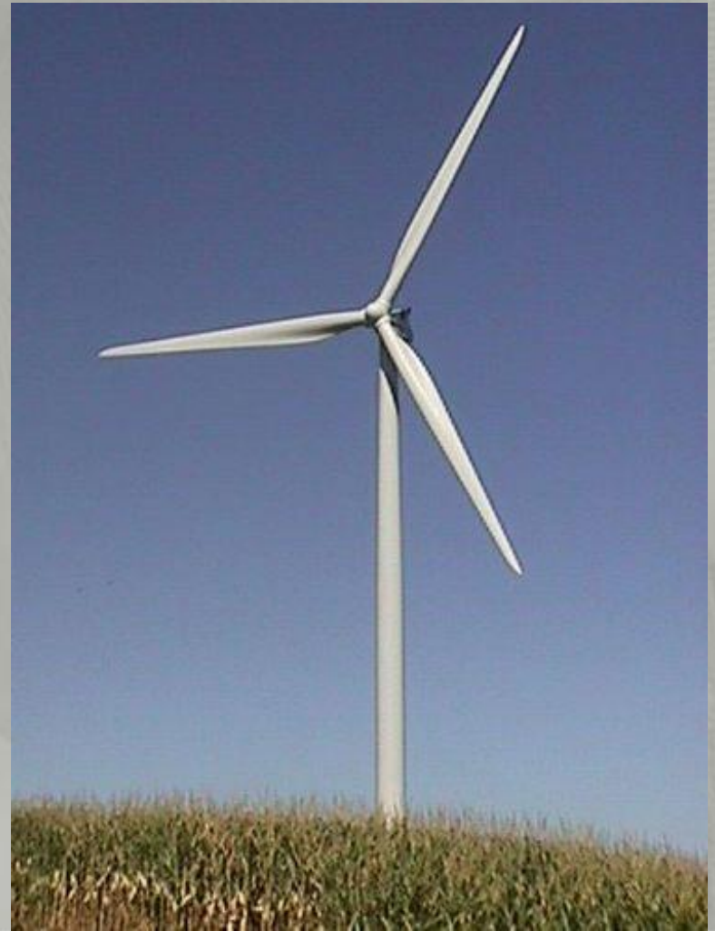
Horizontal Axis Wind Turbine
