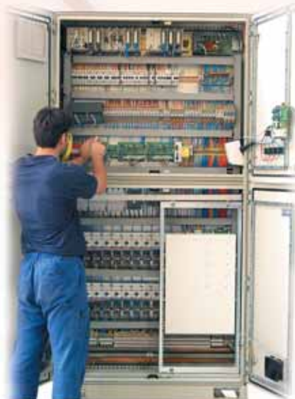
Control electronics and the SITEM A PLC.
