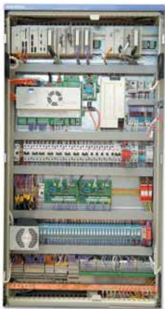
General control cabinet.
