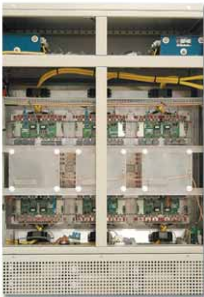
1.5 MW power electronics.
