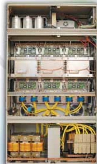
2.5 MW power electronics.
