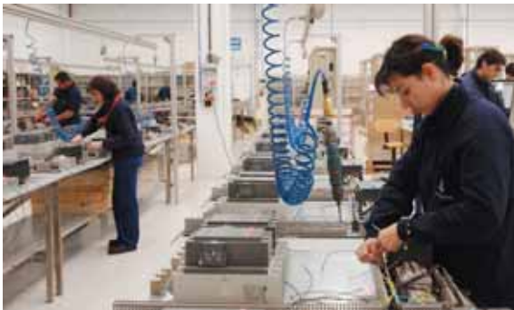
Control cabinet cabling.
